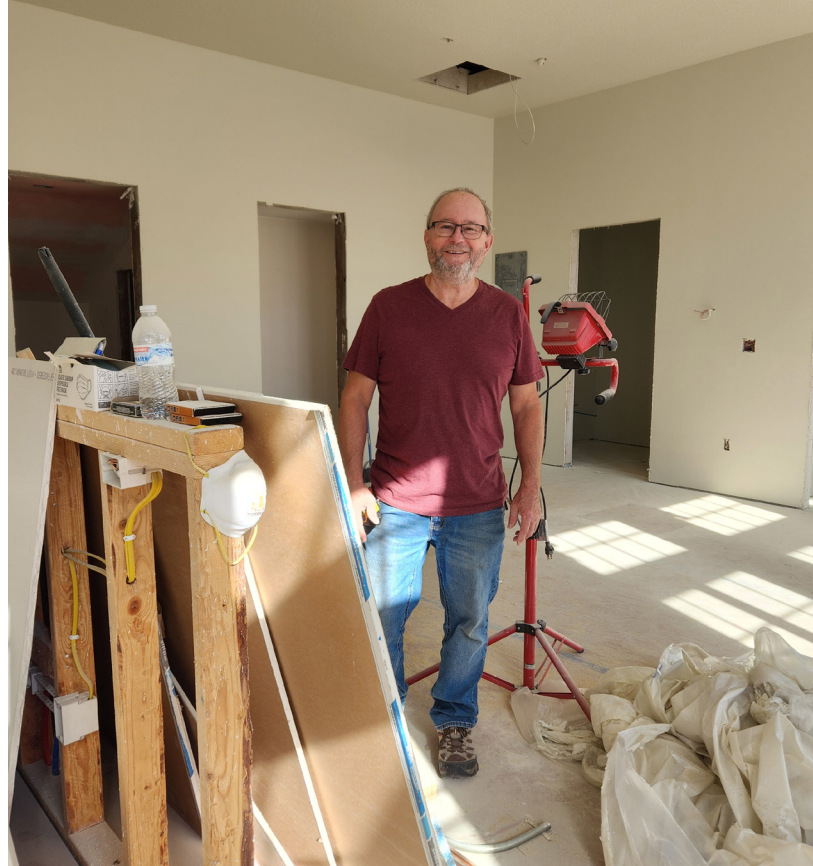
Denny Thompson is using his construction background to help bring the two apartments above the Camelot Theater back to life.
